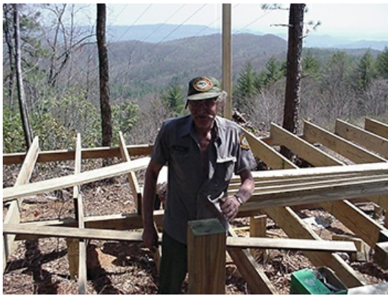
Park staff building a structure with a scenic view behind the work site, Gorges State Park. Photograph, April 11, 2001. North Carolina Division of Parks and Recreation.
