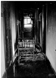
17 July 1936 photo of fire damage in an interior. From the Dunn Area (Lewis White Studio) Photo Collection, PhC.121, North Carolina State Archives, Raleigh, NC, call #: PhC.121-3.
