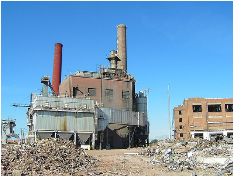
Demolition of Fieldcrest Cannon Mills, Kannapolis, NC, 2004. Image courtesy of Brad Spry.
